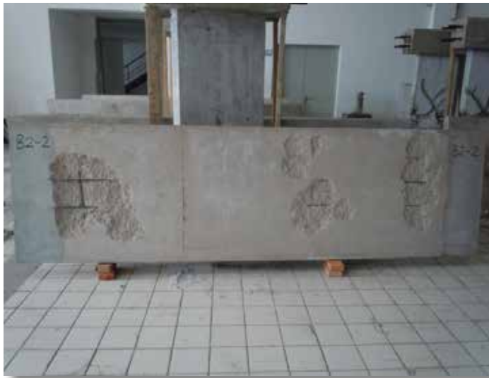
Concrete spalling after fire exposure
