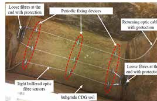
Photo of installation of BOTDA sensing fibre in the subgrade layer Installation method of distributed strain sensing fibre in the subgrade layer
